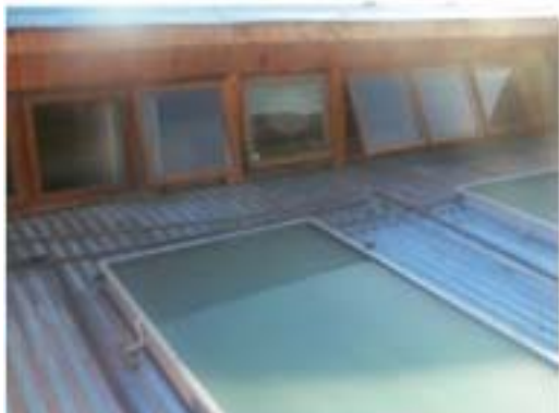
Figure 3: Solar water collectors.
